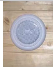
Wall / ceiling speaker
